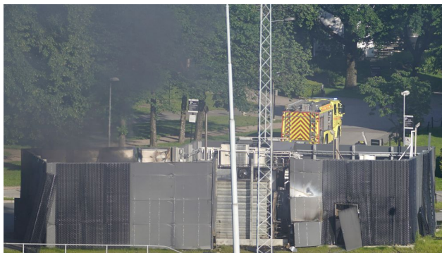
Figure 2. The pressure-wave lifted away the complete roof of the compartment [photo: Heiko Junge / NTB scanpix]
